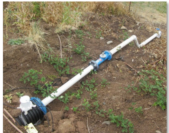
Figure 1: 2" Flow Meter installed on a new pressurized sprinkler system from an Irrigation District.
