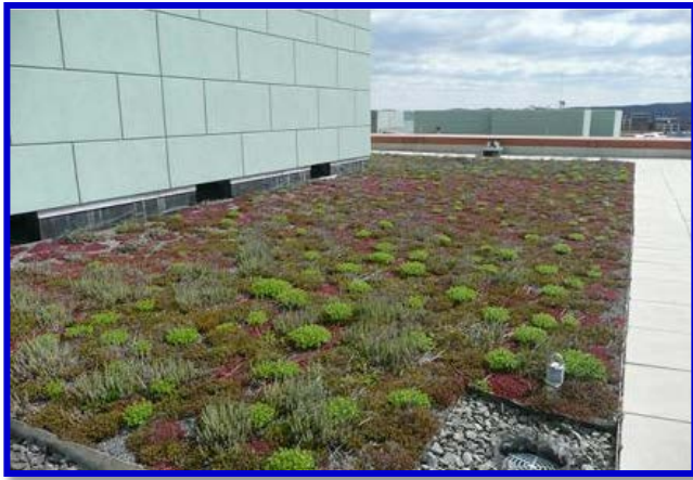
Extensive Green Roof in Washington D.C.
